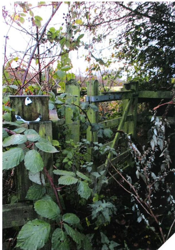
Photograph taken by Mrs V Hourihane, dated 25 th November 2015, showing damaged sign at Rixon Gate end. The gate is overgrown, but is not wired shut at this time.
